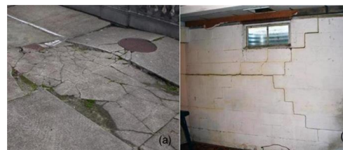
Fig. 1. Cracks in (a) pavements and (b) buildings
